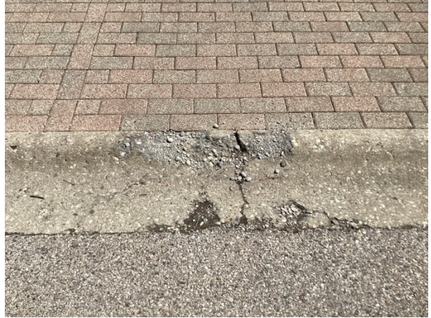
Damaged curb and gutter at Hampton Court
