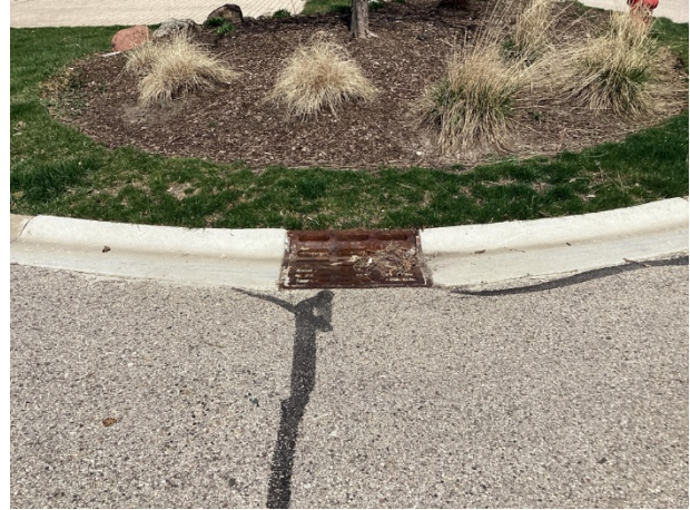
Previous replacement of the surrounding concrete curb and gutter at Hampton Court
