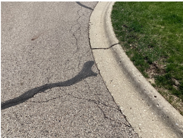
Minor edge deterioration at Narragansett Court
