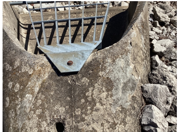
Minor concrete deterioration at the main inlet structure
