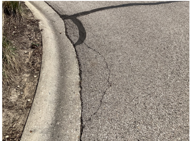
Minor edge deterioration at Narragansett Court
