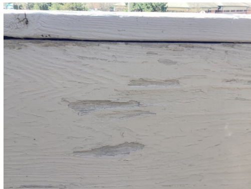
Wood deterioration at back of signage
