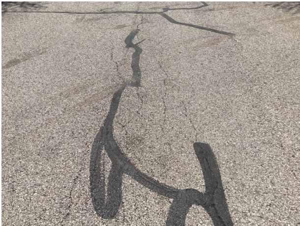
Recent crack repairs and hairline cracks at Hampton Court
