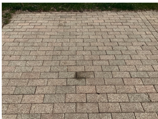
Stained pavers at Hampton Court
