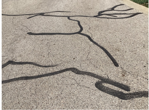
Recent crack repairs and hairline cracks at Sedgewick Court
