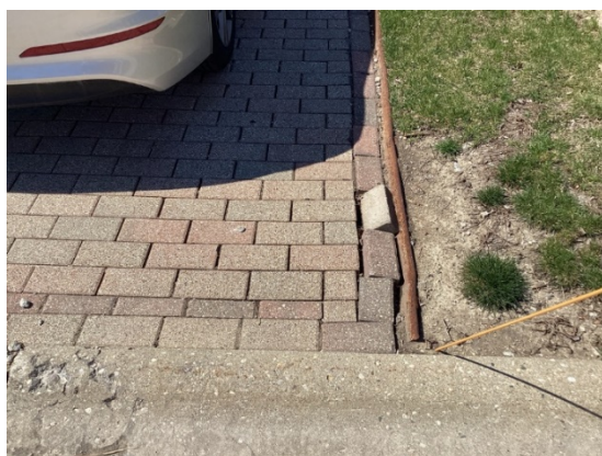
Loose pavers at Sherbrook Court
