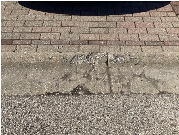
Damaged curb and gutter at Sherbrook Court
