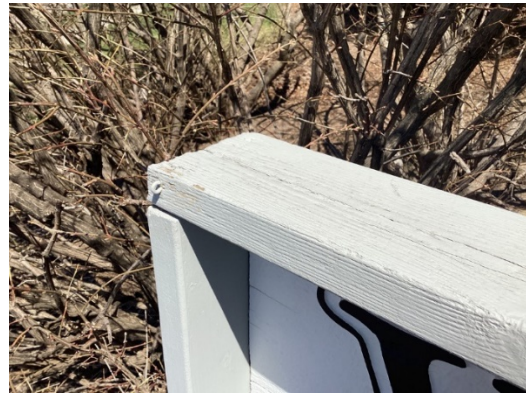
Weathered wood trim
