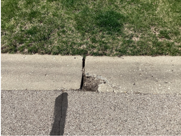
Damaged curb and gutter at Hampton Court
