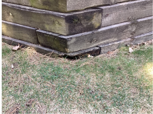
Rotted wood along bottom of wall
