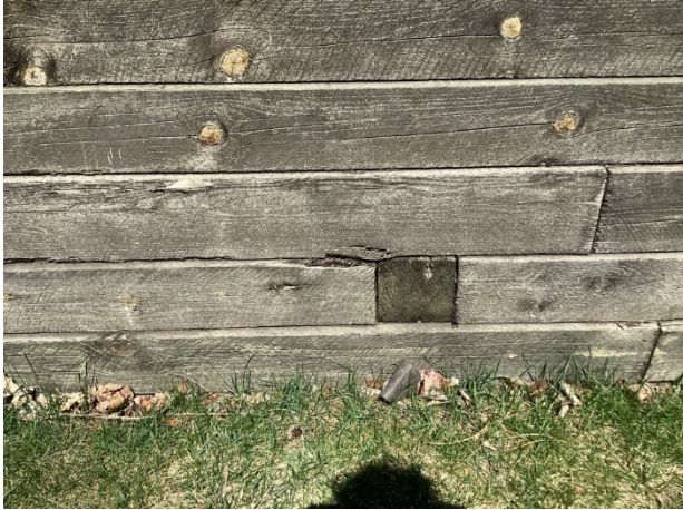
Minor wood deterioration near deadman
