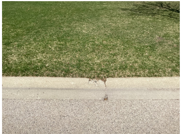
Damaged curb and gutter at Norwich Court
