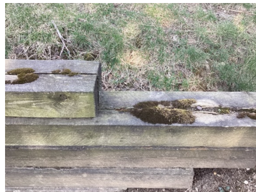
Rotted wood along top course of wall
