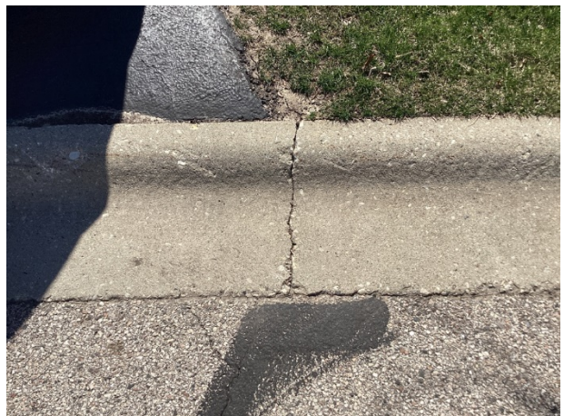
Curb and gutter crack at Norwich Court
