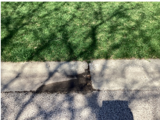
Damaged curb and gutter at Norwich Court
