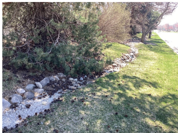
Erosion and insufficient gravel coverage
